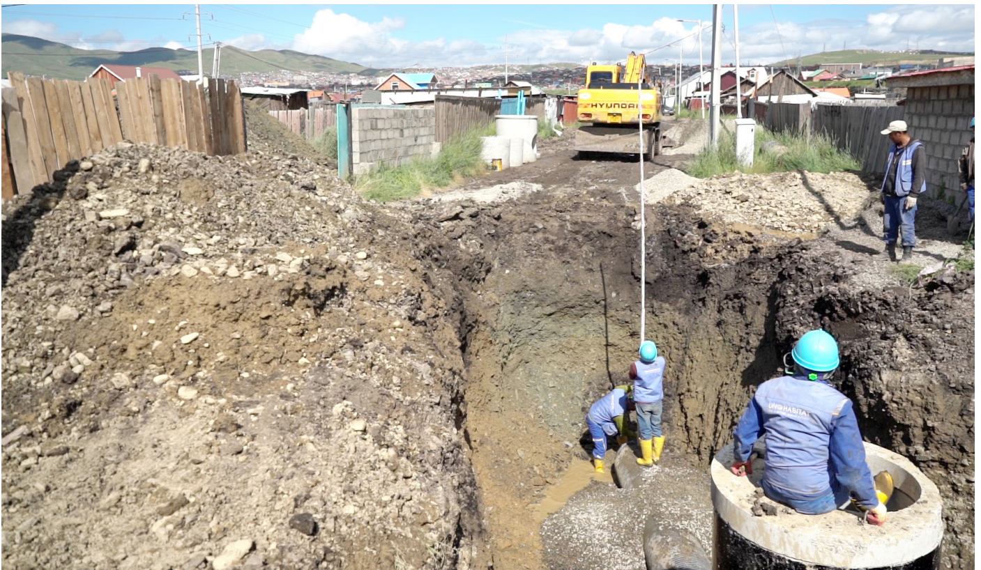
Flood protection facility construction in the suburb of Ulaanbaatar City. © UN-Habitat Mongolia
